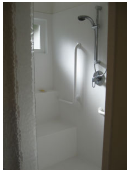
This seamless shower features a bench, window coving, handrails and a hand-held spray unit.
